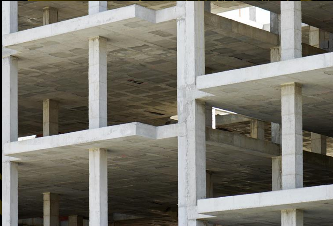
Concrete Flat Slab
