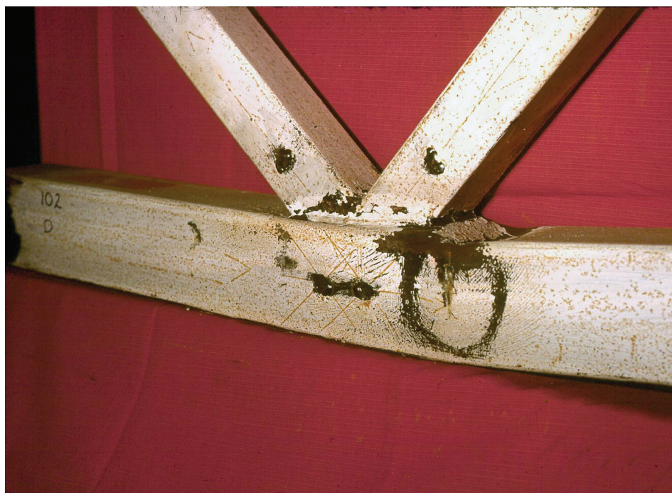
Fig. 2-17. Local buckling of chord due to uneven load distribution.
