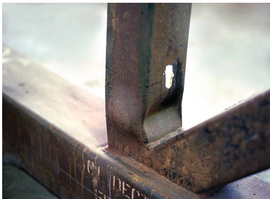
Fig. 2-13. Local yielding of a branch in compression due to uneven load distribution.
