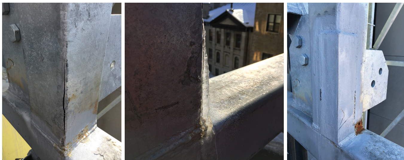
(a) Longitudinal cracking in a cold-formed corner with low ductility
