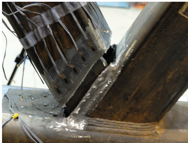
Fig. 3-17. Typical fillet weld and PJP groove weld fracture for an HSS-to-HSS overlapped K-connection.
