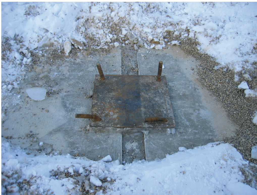
Fig. 4-17. Anchor rods run over by a crane.
